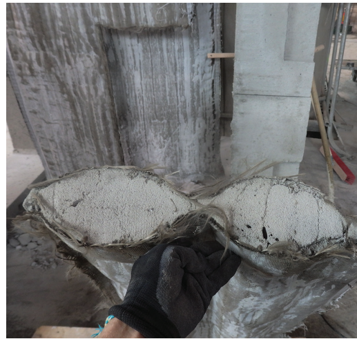
FIG. 18 In the background, large-format basalt fabric, foamed with cement foam, height 3.80 m, section of the element in front
