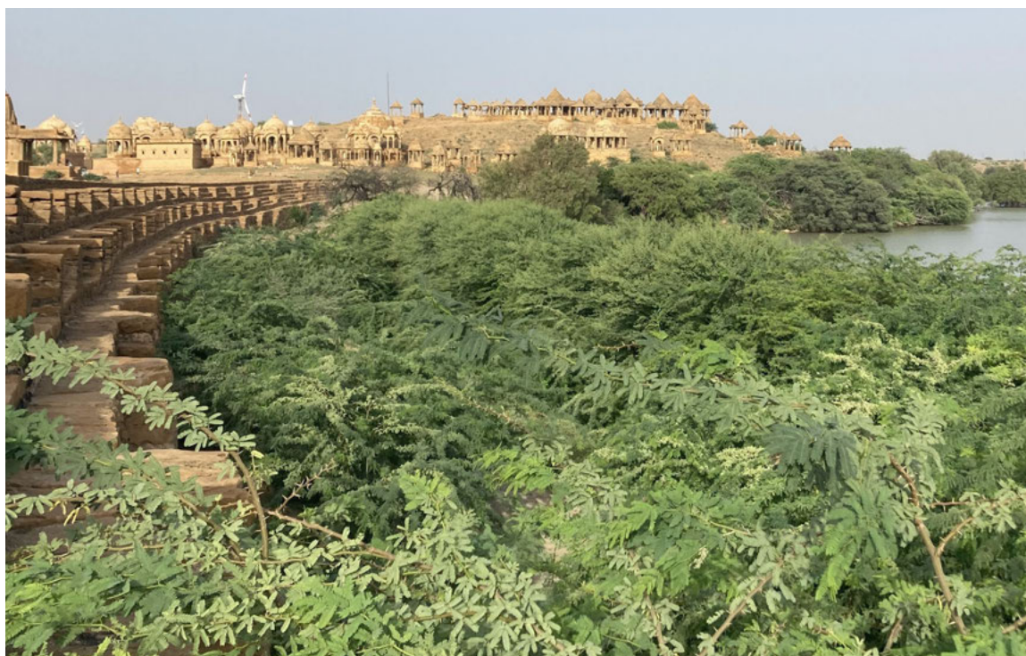
^ Fig. 4 Stone embankment overrun by vegetation at the Bada Bagh Khadeen (Source: Pierantonio La Vena, 2023).
