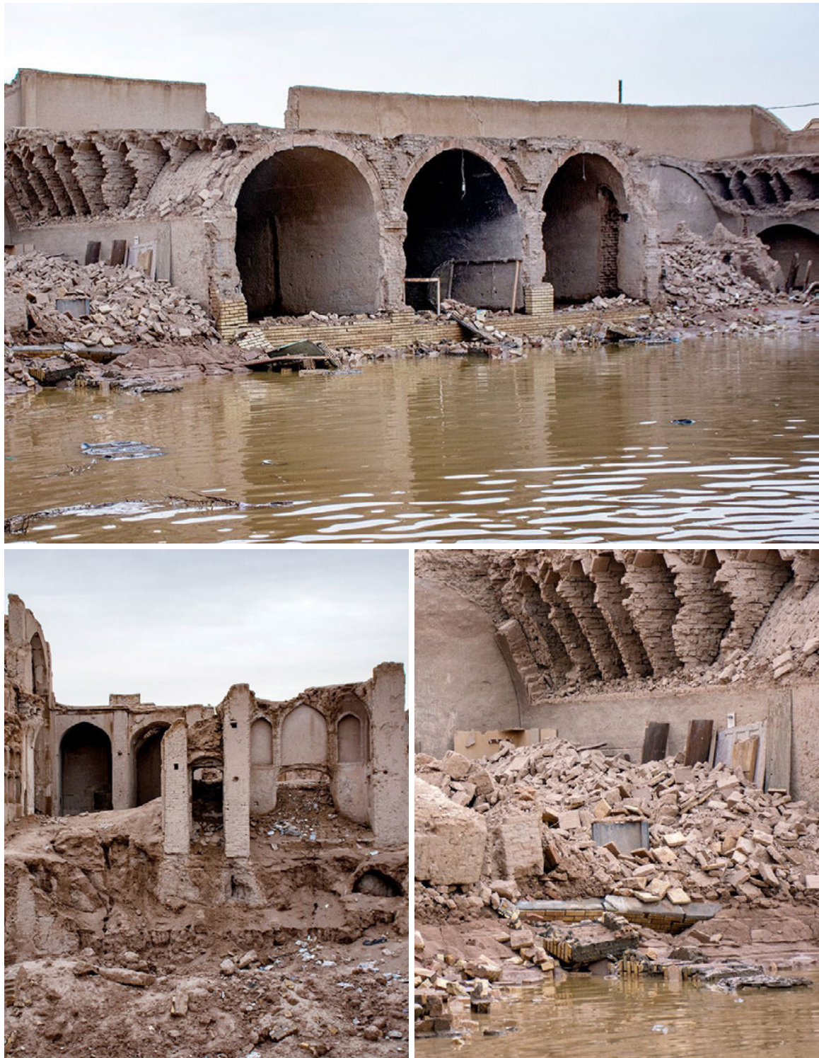
^ Fig. 6 Destruction of historical fabric due to flooding, Yazd, Iran, 2022 (Source: Majid Jahrahi).
