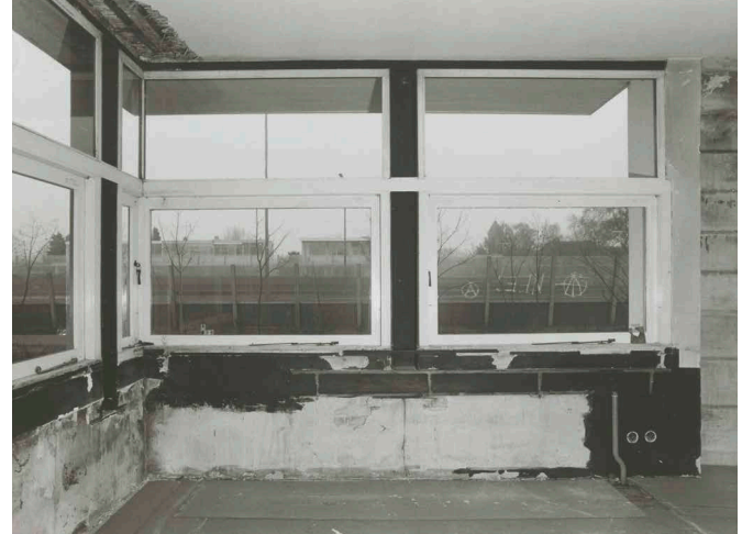
FIG. 3.4 The corner window during the restoration, with a view of the viaduct and the houses on Erasmuslaan
