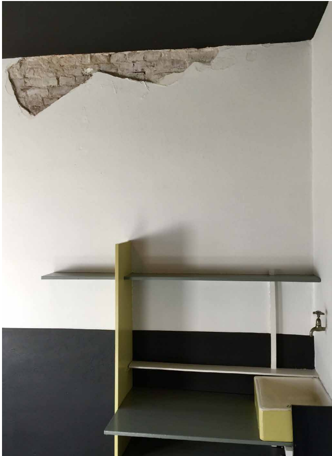
FIG. 3.13 The plasterwork at the top of the south wall of the study was damaged and came loose in October 2016
