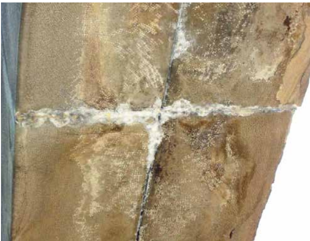
FIG. 3.1 Efflorescence of stone wall (Stefanović, 2010)
