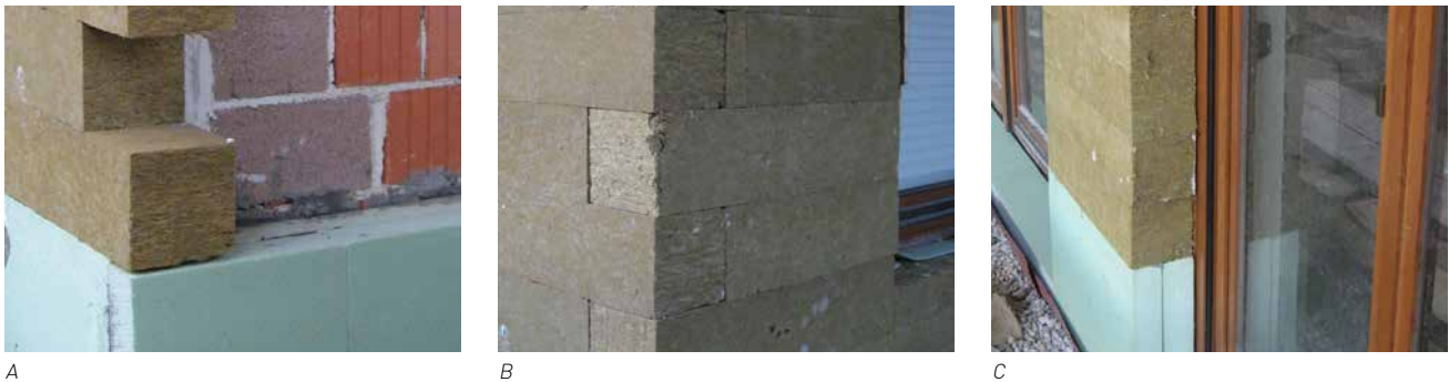
FIG. 4.1 A+B+C: A massive wall – brick with external mineral wool and XPS thermal insulation
